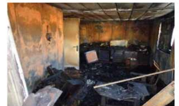
Damage to the Master's Cabin and Office
