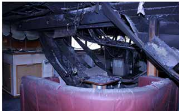
Fire occurred in the Bridge ceiling/void
