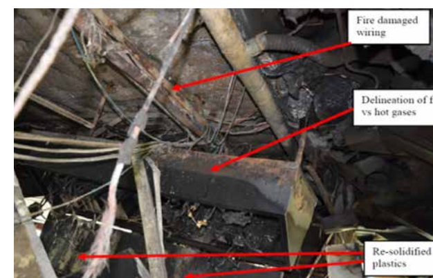
Where the fire started
