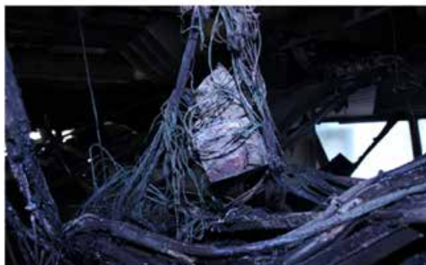
Damaged wiring and circuit board which was fitted to the plywood board.
