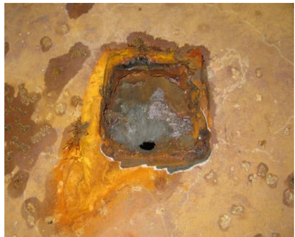
Example of the effects of galvanic corrosion
