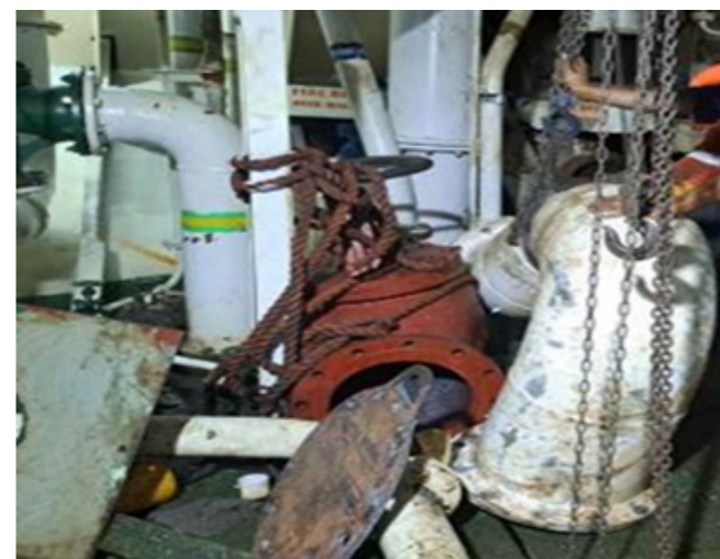
Corroded pipes, with seawater valves dismantled for repair / replacement
