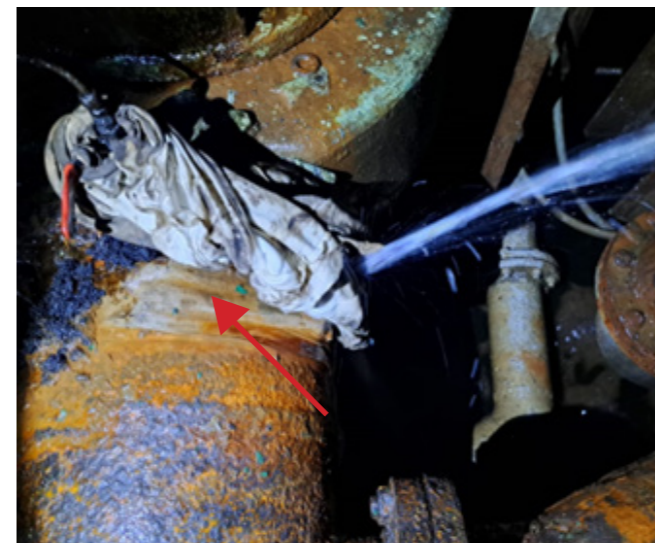
Leakage from corroded pipe - previously 'repaired' by soft patching (red arrow)
