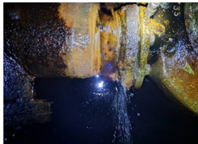
Leakage from seawater pump pipe flange welding due to corrosion
