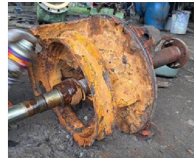
The pump cover and pump housing were found to be heavily corroded
