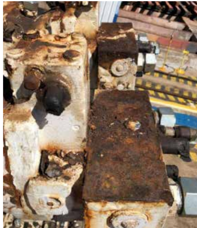
The effects of poor maintenance on hydraulic components
