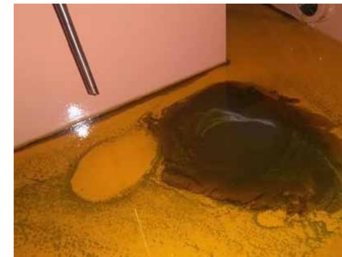
Sediments and impurities in power pack oil tank
