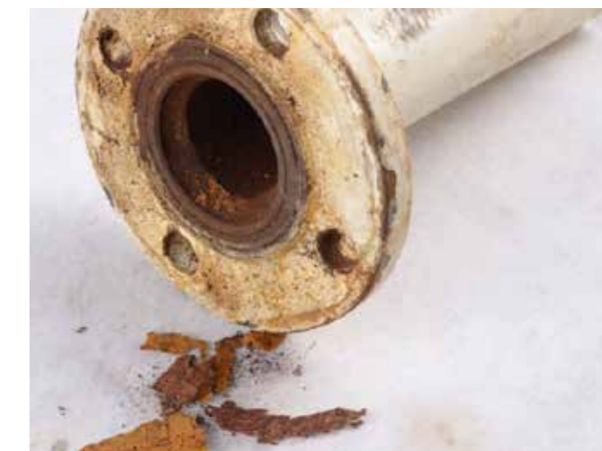
Corroded pipe, not up to Class standard, with debris
