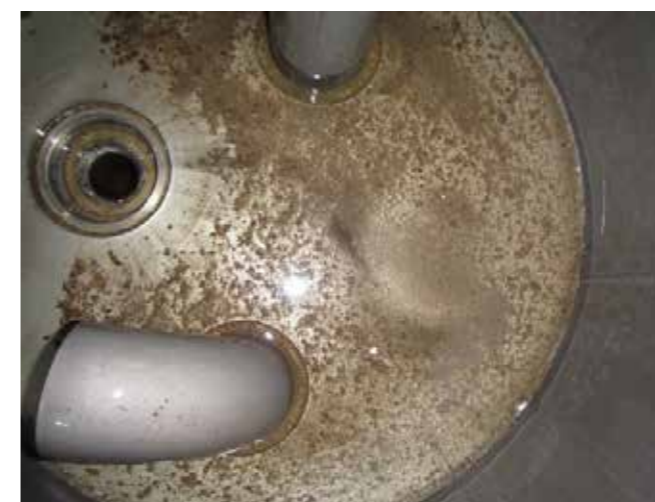
Debris in the bottom of an oil gravity tank
