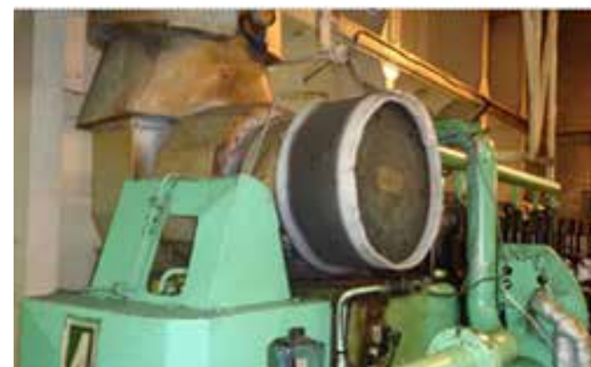
Such polyester filter material is frequently used, incorrectly, as a substitute air filter material on turbochargers
